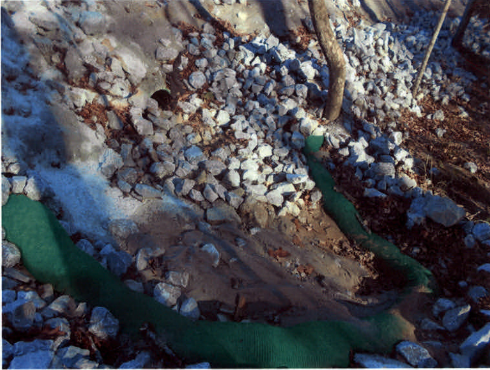
Sediment Trap Discharge Point
